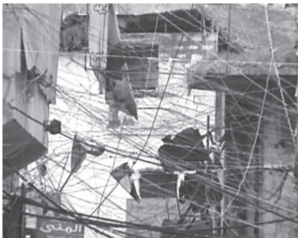
Fig. 16 Shatila camp: A web of cables covers narrow streets.
